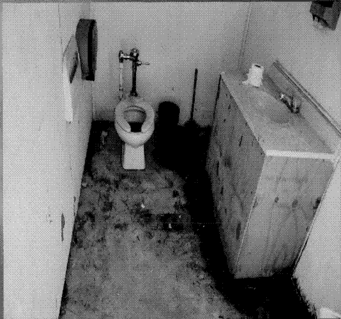
Plywood under sink has water damage and starting to rot
