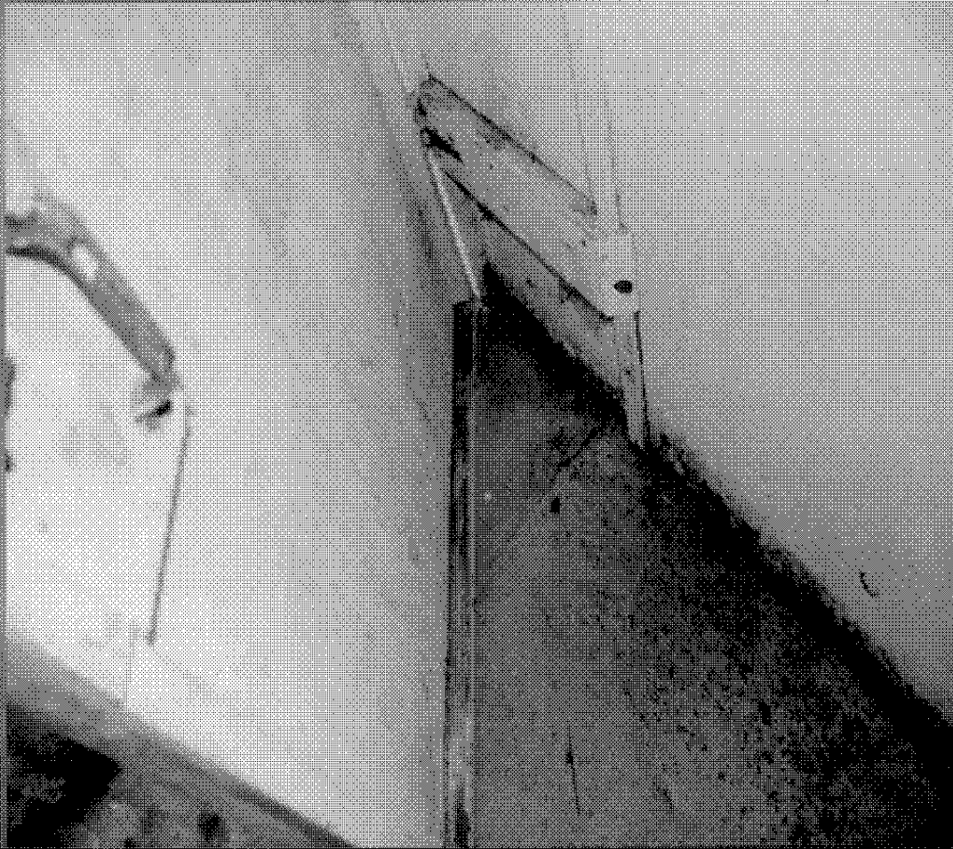
More water damage behind the door, doors seam to be in good shape and just require clean up and repaint
