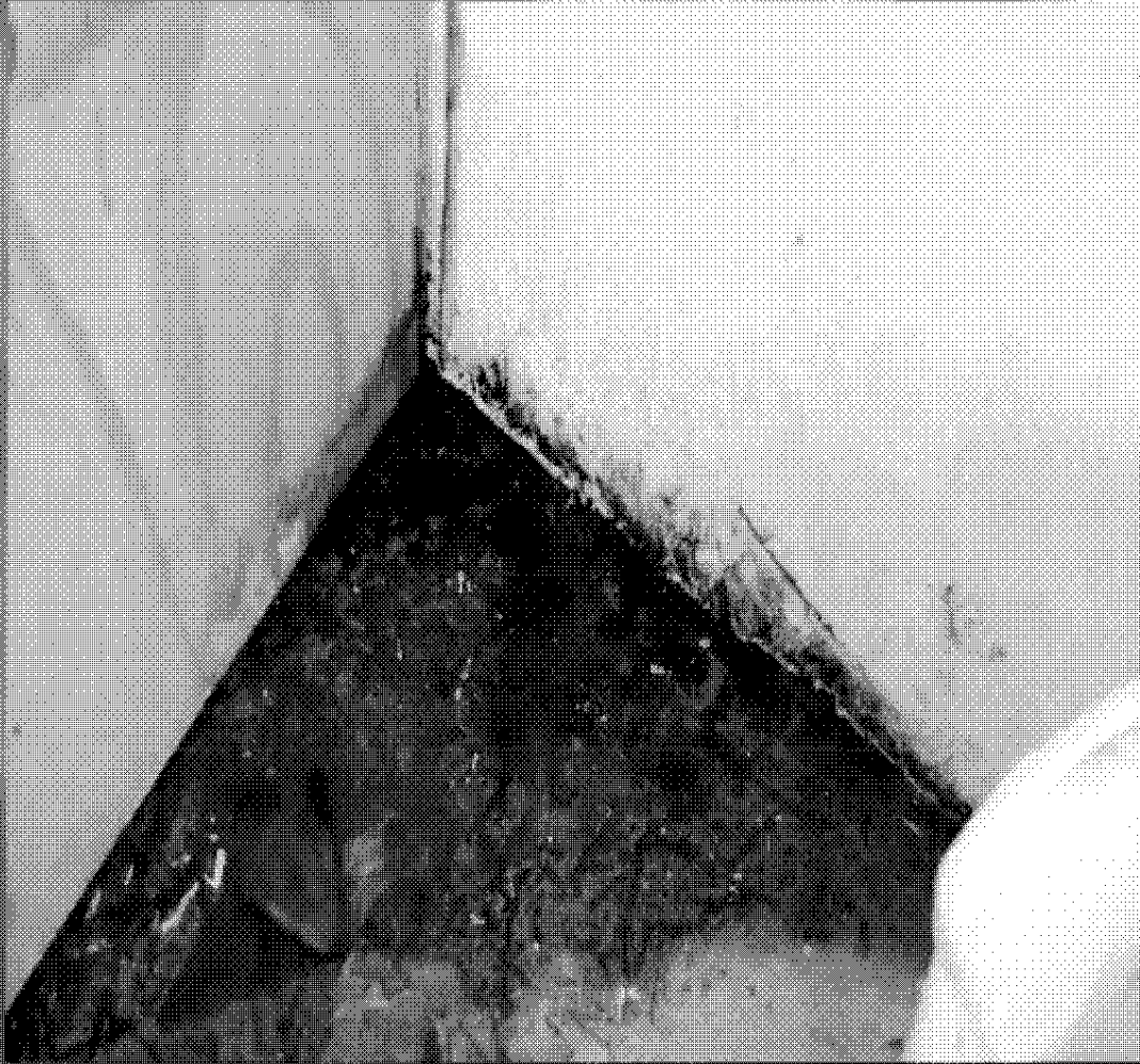
Water damage on plywood and wafer board is coming apart due to water damage
