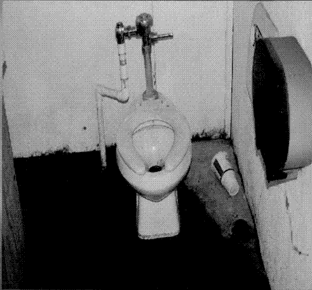
Fixture all seem to be in good shape and plan to re-use
