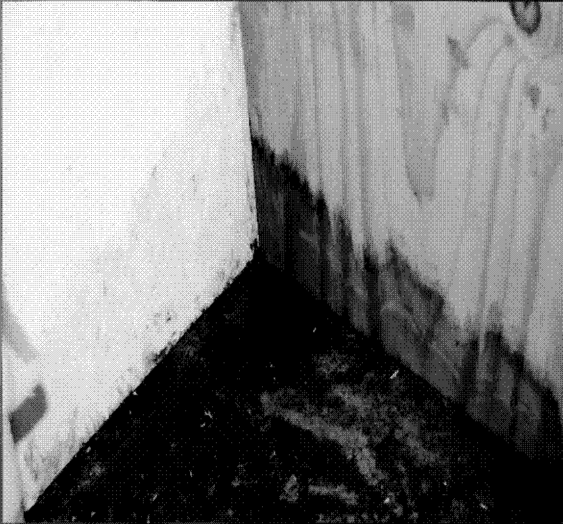
Water damage to the sink cabinet and interior walls in both bathrooms
